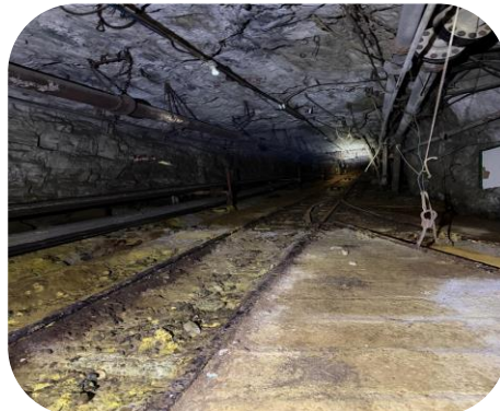
Cable belt conveyor to 850 level
